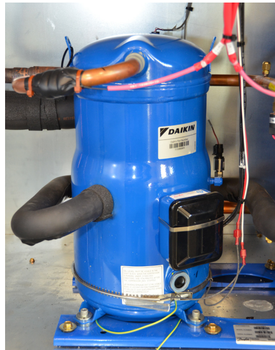
Figure 32: Compressor Suction and Discharge on DPS 025–028 units
